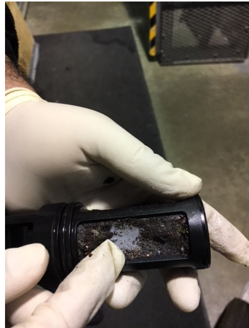
Figure 5-15. Clogged Pump Strainer
