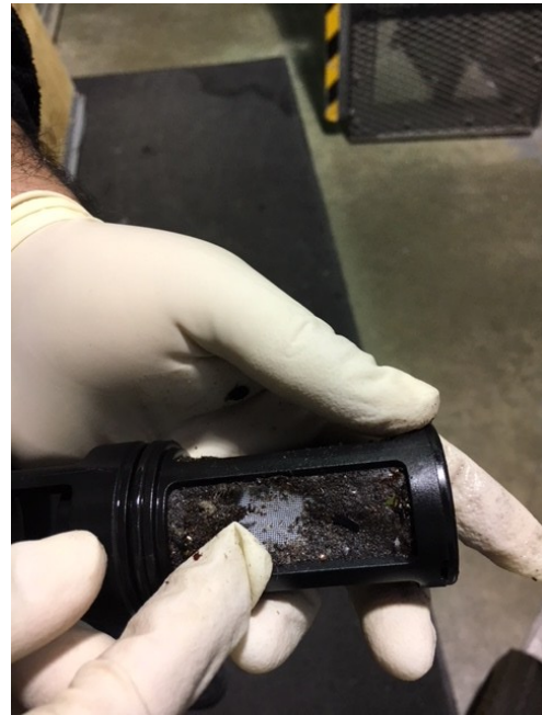
Figure 5-15. Clogged Pump Strainer
